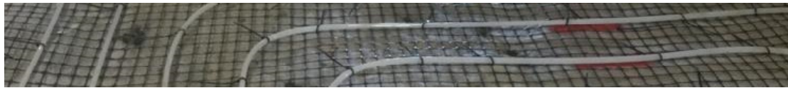
UNDERFLOOR HEATING (OPTIONAL) ATTACHED TO GEOGRID USING CABLE TIES AND CLIP RAILS BY HEATING CONTRACTOR ↑
